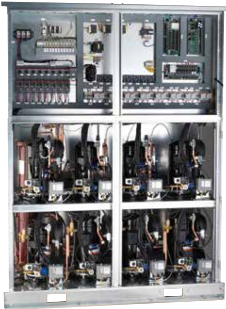
CENTRALIZED PIPING AND ELECTRICAL
