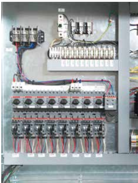
ELECTRICAL/ CONTROL PANELS
